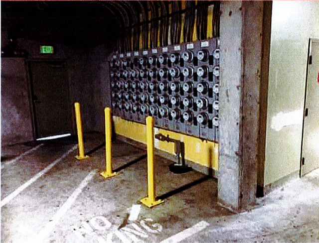
7 - ELECTRIC SERVICE METERS
