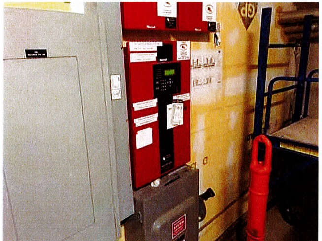
22 - MULTIPLEX FIRE ALARM PANEL
