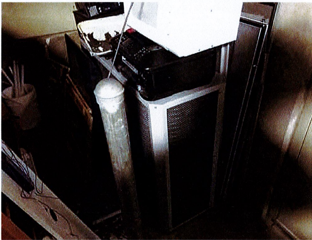
27 - SPLIT SYSTEM DUCTLESS
