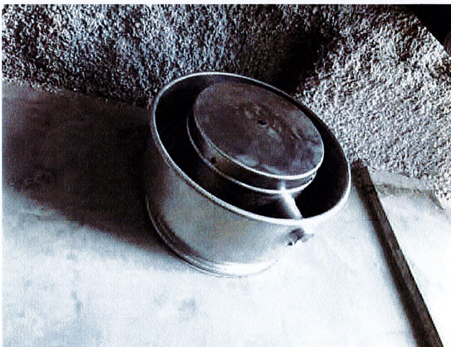
29 - WALL-MOUNTED EXHAUST FAN
