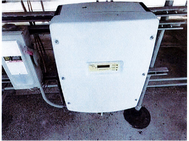
46 - SOLAR POWER, INVERTER
