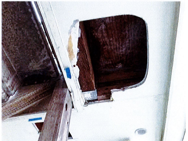
48 - WATER DAMAGED WOOD FROM WATER INTRUSION
