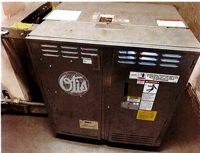
23 - HYDRAULIC ELEVATOR EQUIPMENT
